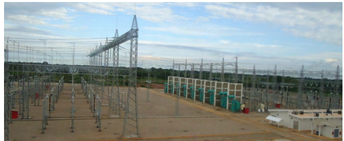
Fig. 1. View of the Tabasco 400/230 kV substation.
