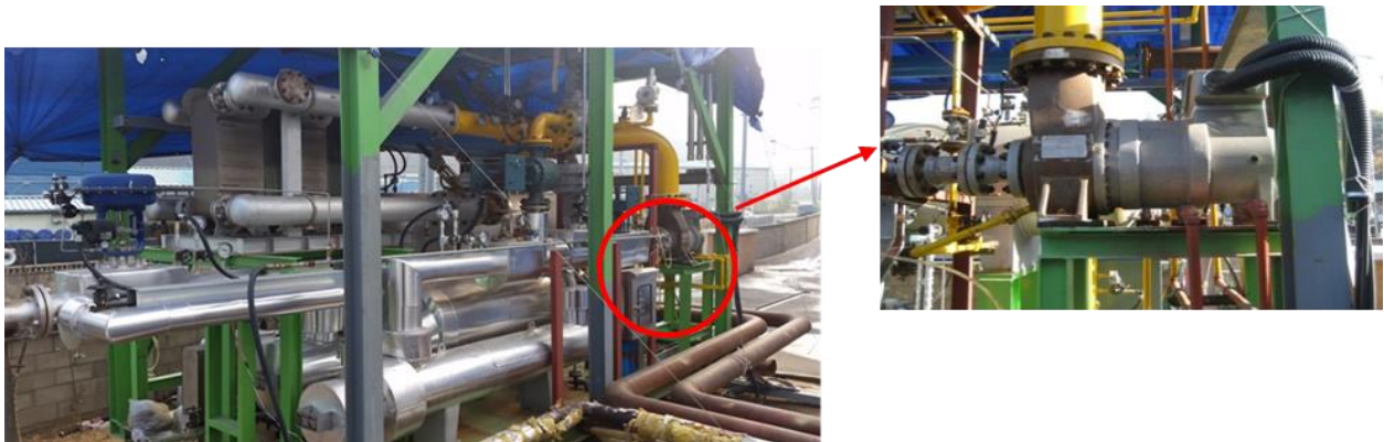
Figure 12. Mounted example of a single 300 kWe ORC module.
