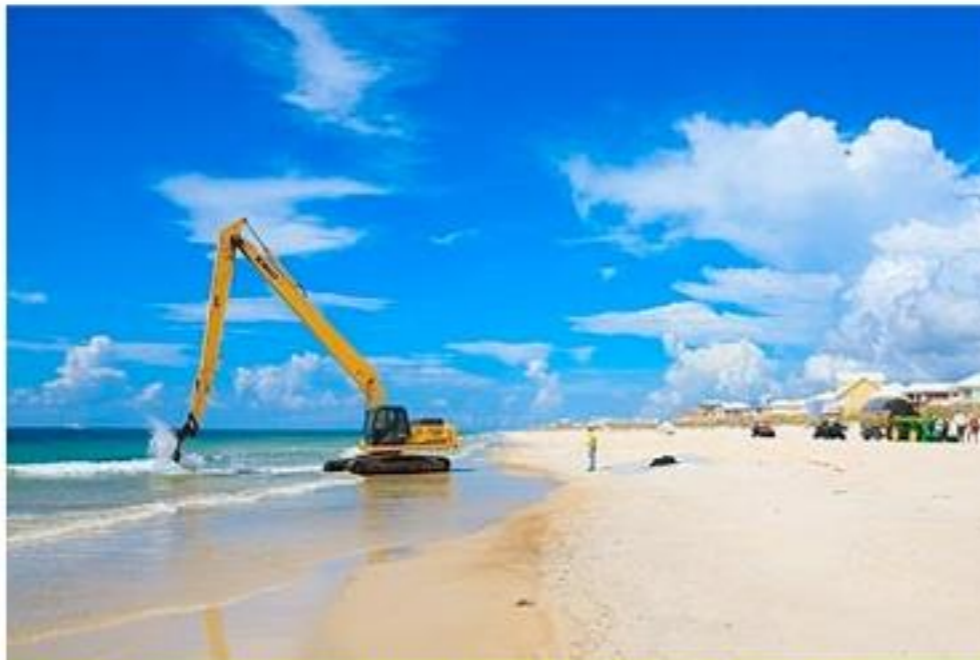
A large excavator is used to pull buried snare boom from the shoreline of Gulf Shores, AL on September 11, 2010
