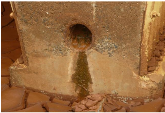
Figure 4 Cracks across the foundation level CSP
