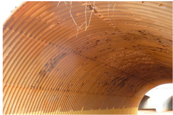
Figure 5 Advanced corrosion to CSP
