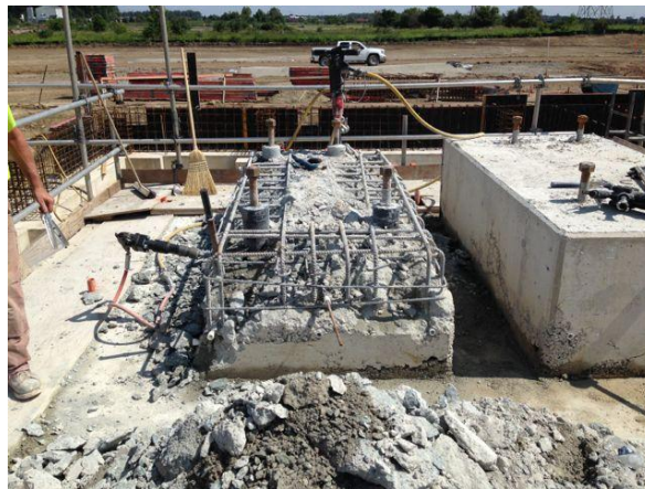
Figure 17: Parkway “C” compressor pedestal following jackhammer removal of honeycombed concrete
