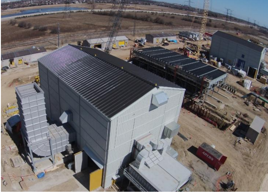
Figure 12: Parkway C and D Compressor Buildings
