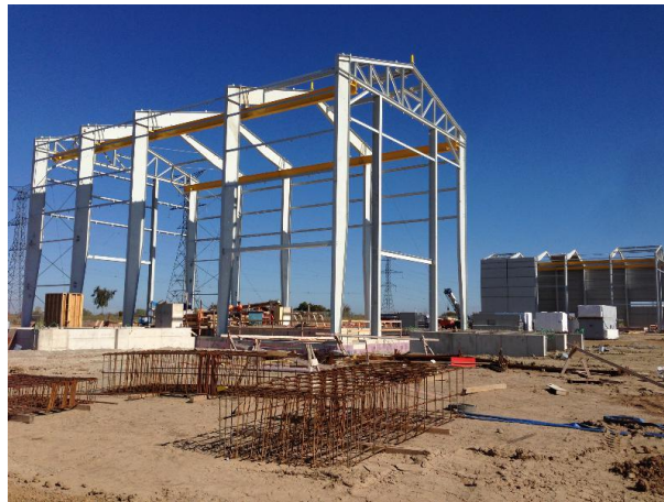
Figure 18: Parkway “C” compressor building structure in foreground; partially enclosed Parkway “D” compressor building in background
