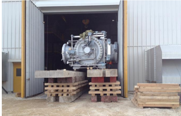
Figure 6: Photo of the Parkway “C” Compressor During Installation
