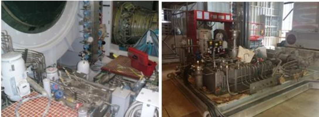
Figure 8: On Skid Gas Generator Lube Oil Console Design and New Off Skid Design
