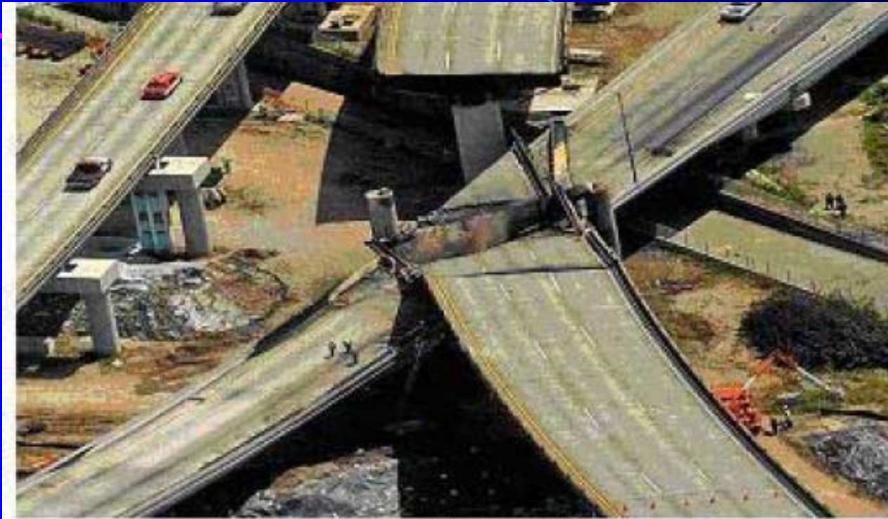
View of damage from above
