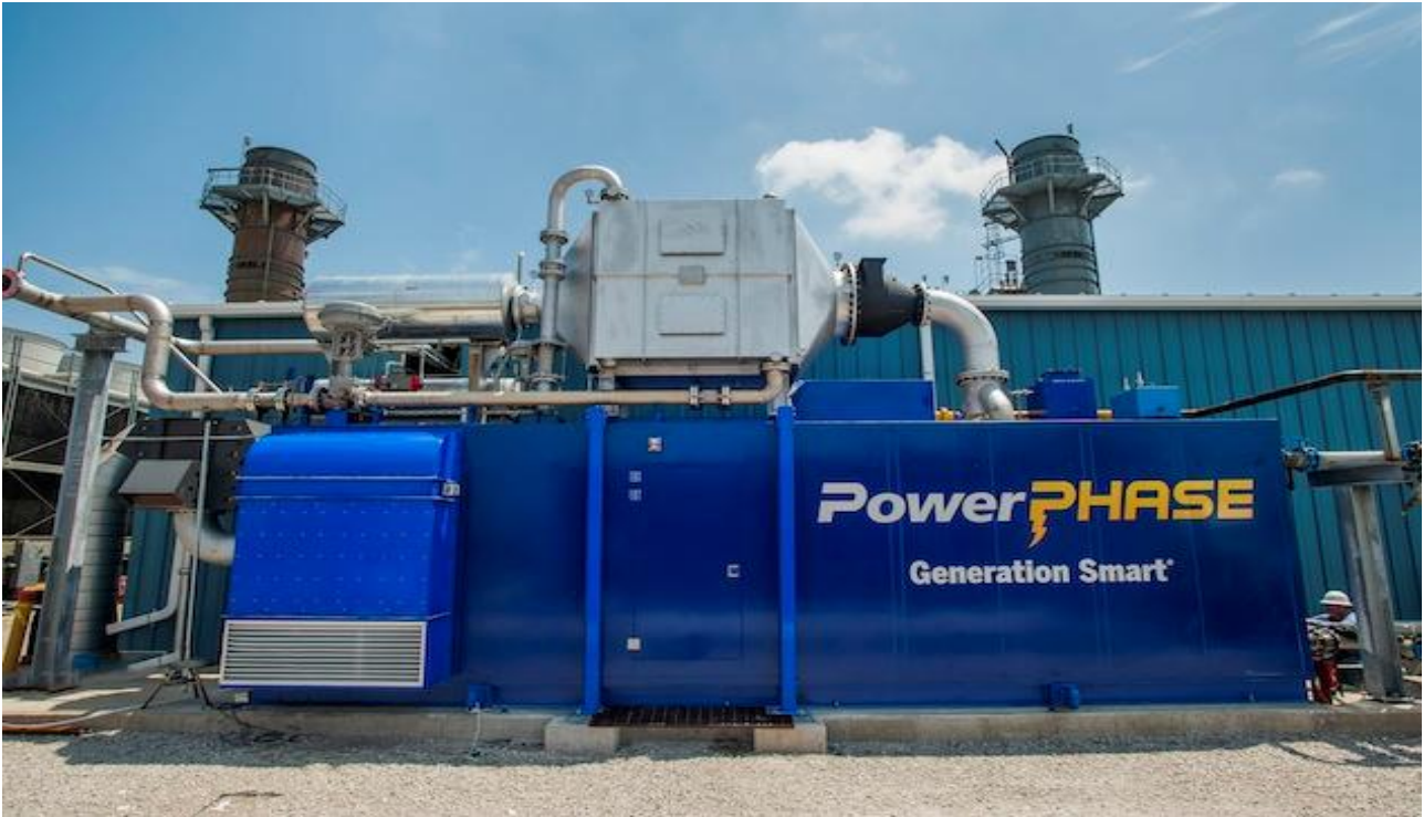
Figure 2: TPM installed at the Morris Cogeneration 3x1 Combined Cycle Plant
