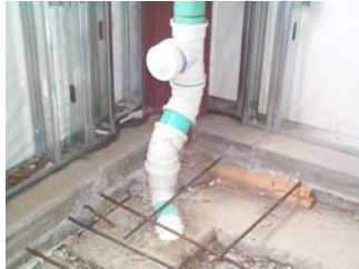
PVC Ventilation Pipe Riser
