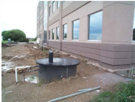
Sump for drainage from methane gathering system
