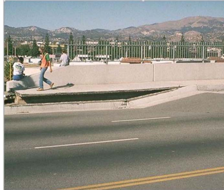
Figure 63: Settlement of the approach slab ( NYSDOT )
