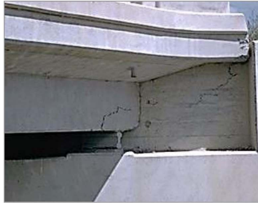
Figure 77: Superstructure spalled at bearing location ( NISEE )
