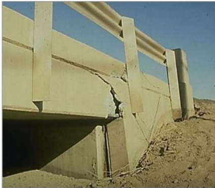
Figure 86: Cracking and rotation of wingwall (NISEE)
