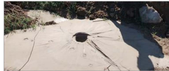
Figure 102: Liquefaction sand boil ACTION: Report findings immediately and request Stage 2 Inspection. Close bridge when sand boils are present near substructure.
