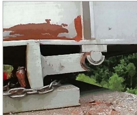
Figure 78: Rocker bearing failure ( NISEE )
