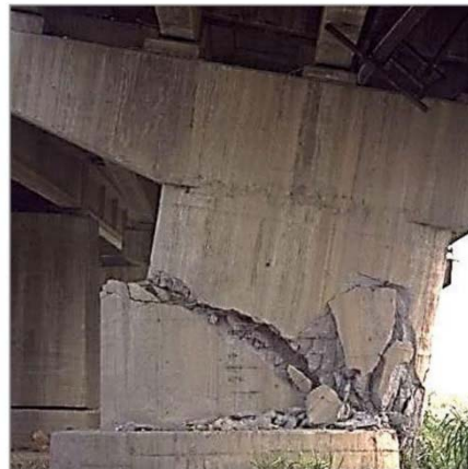
Figure 92: Full collapse of pier (NISEE)
