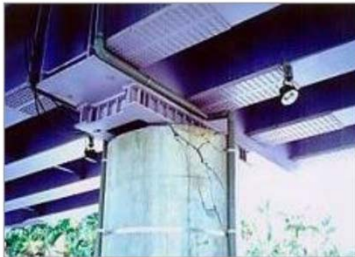
Figure 95: Compression failure on the top of concrete bridge pier ( INDOT ) ACTION: Report findings immediately and request Stage 2 Inspection.
