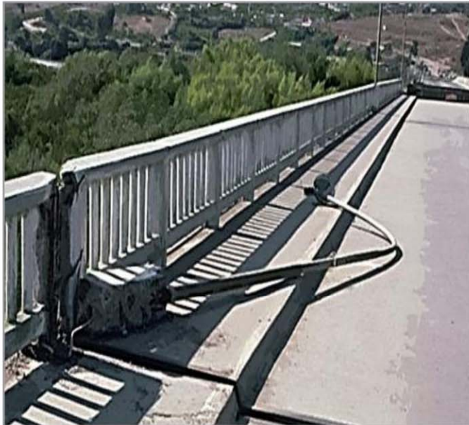
Figure 71: Collapse of street lighting elements ( NISEE )
