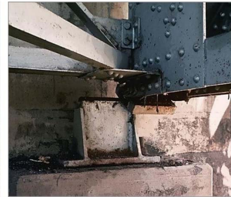
Figure 79: Failure of bearing, complete lateral displacement ( NISEE )
