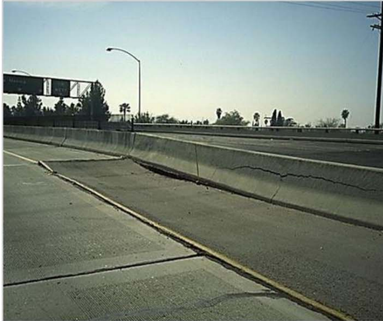
Figure 62: Approach slab settlement and cracking of the concrete barrier ( NISEE )
