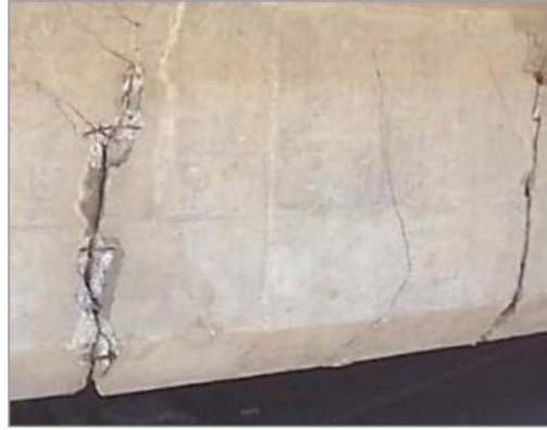
Figure 74: Cracking in web of concrete beams ( NYSDOT )
