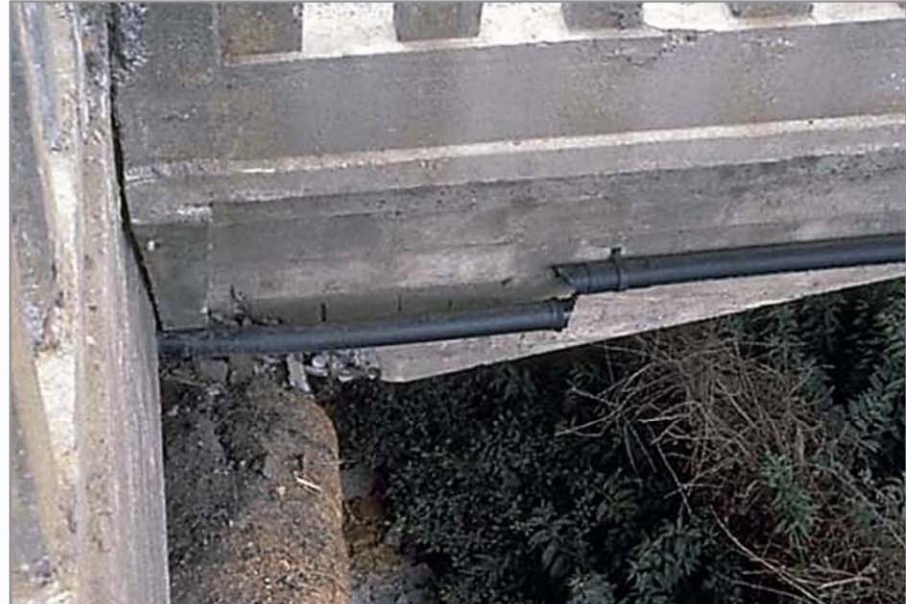
Figure 72: Broken pipeline conduit ( NISEE )
