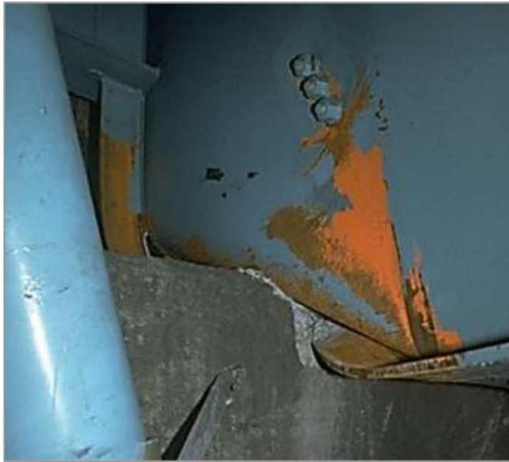
Figure 76: Damage to beam caused by movement of the structure ( NISEE )
