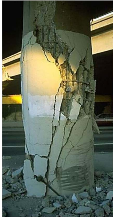
Figure 96: Confinement failure in single column ( NISEE ) ACTION: Close bridge. Report findings immediately and request Stage 2 Inspection.
