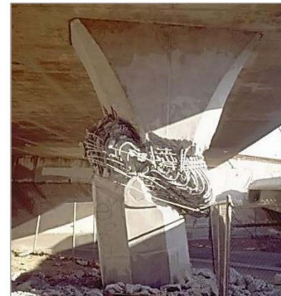
Figure 93: Failure of column (NISEE)
