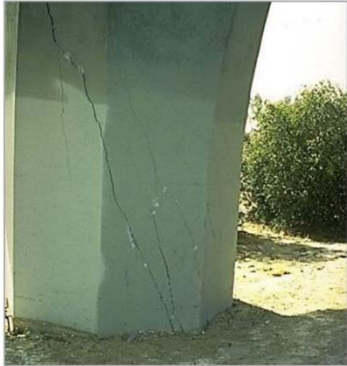
Figure 94: Shear cracks in column ( NISEE ) ACTION: Bridge remains open. Report findings immediately and request Stage 2 Inspection.
