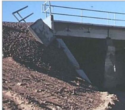
Figure 87: Wingwall released from superstructure after earthquake tremors (NISEE)
