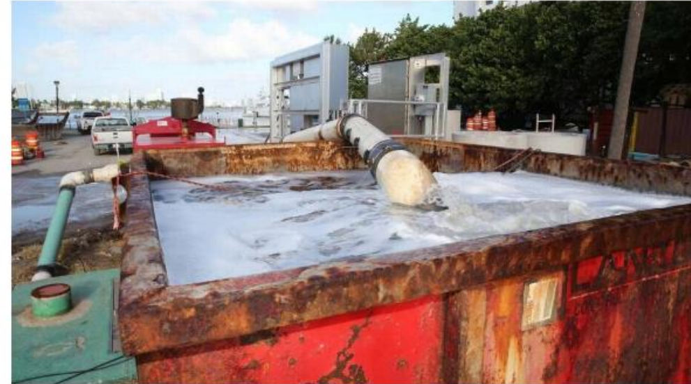
An anti-flooding water pump roars at full capacity at Maurice Gibb Park in the 1800 block of Purdy Ave. in Miami Beach due to the beginning of King Tide last October. C.M. GUERRERO - cmguerrero@elnuevoherald.com
