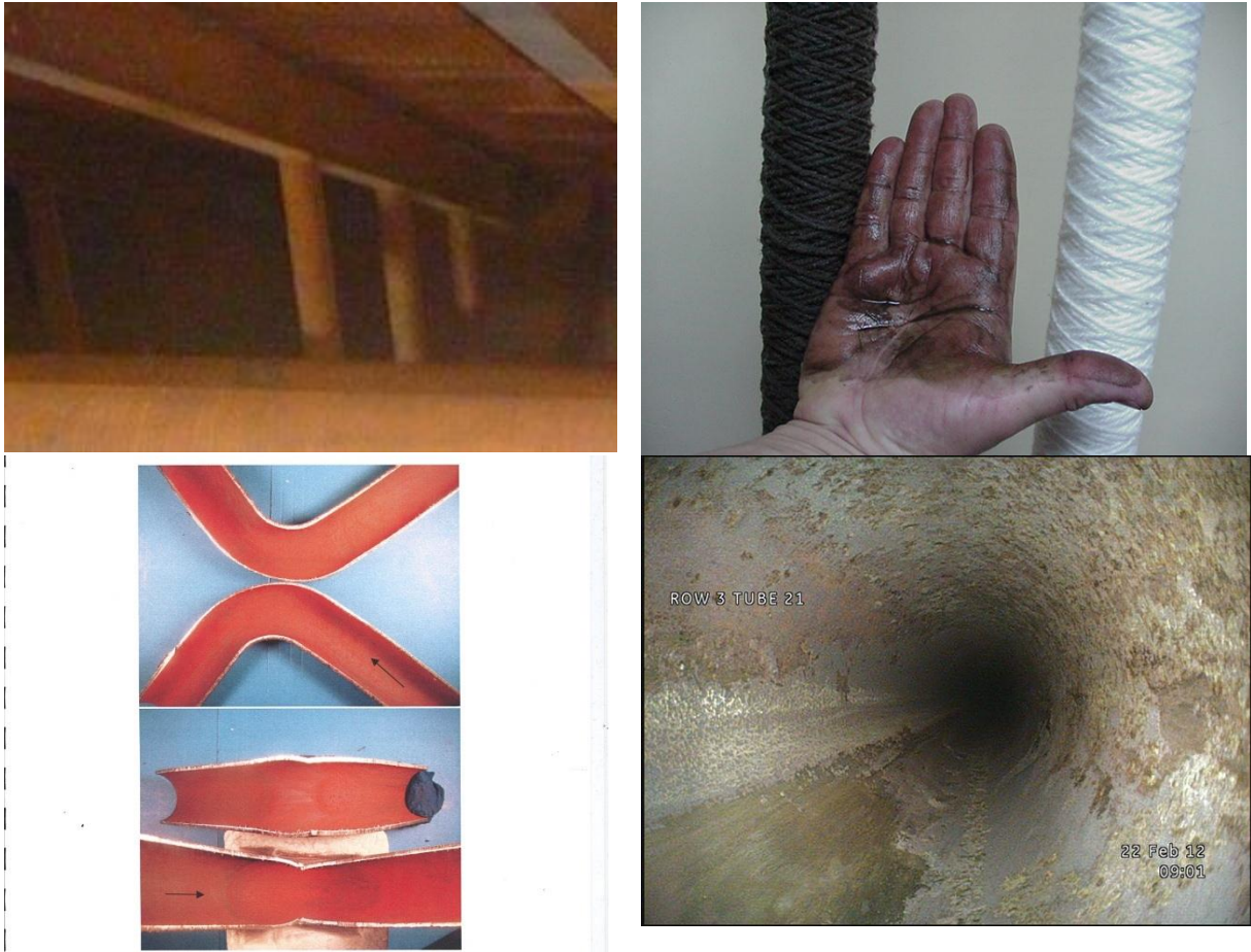
Figure 4: Flash Rusting (Hematite Blooming) Inside Condenser Hotwell (Top Left), Fouled Polisher Element due to Iron Transport from Flash Rusting (Top Right), OTSG Boiler Tubes Coated with Transported Iron Oxide (Bottom Left), OTSG Boiler Tube Showing Iron-Oxide Deposits due to High TDS
