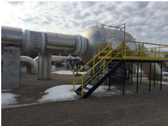
Figure 2: Acoustical lagging on 1 metre diameter suction piping (and scrubber) of a gas turbine-powered natural gas compressor plant.
