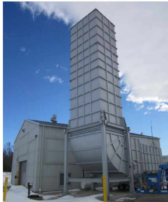
Figure 1: An industrial gas turbine exhaust silencer.
