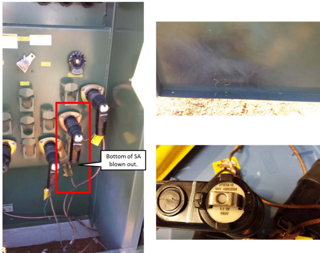
Figure 9 Left: Damage to surge arrestor that did not have sufficiently high MCOV rating. Top right: Damage to transformer door. Bottom right: MCOV rating show 8.4 kV.
