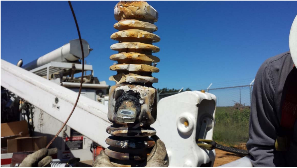
Figure 7 Damage to fuse insulator.
