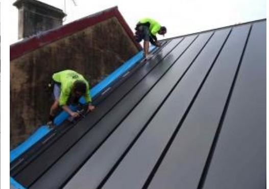
BlueScope BIPVC world-1 st integrated solar energy / cooling and heating roof system in Glebe
