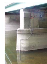
Scour Monitoring Device
