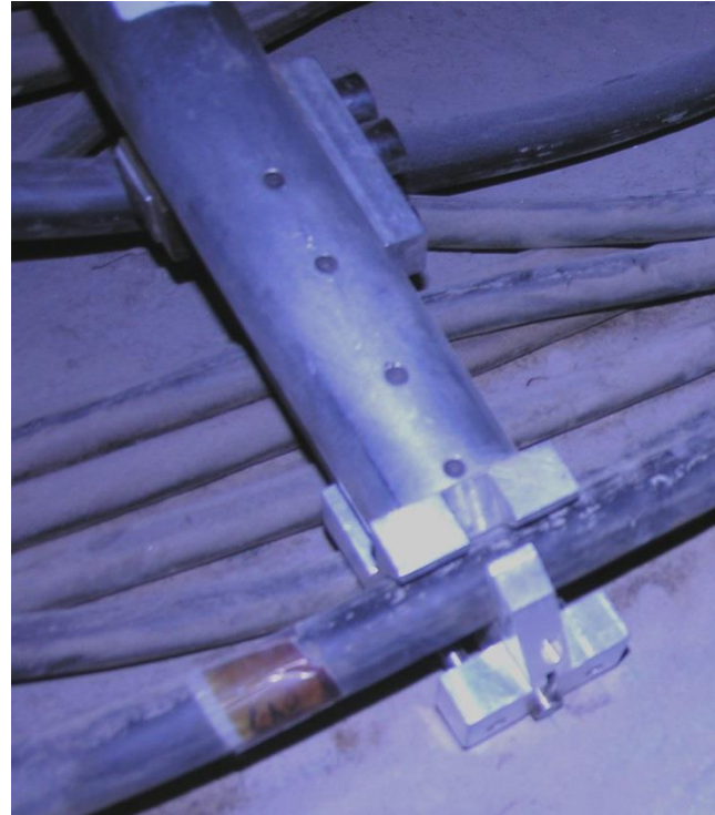
The Indenter Tool in a cable tray as used in the field
