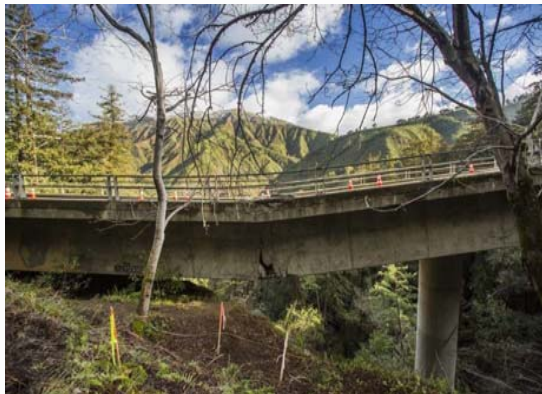
Damaged Pfeiffer Canyon Bridge
