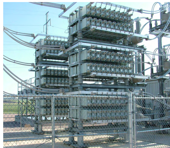
Fig. 14. Capacitor bank with sun on right side
