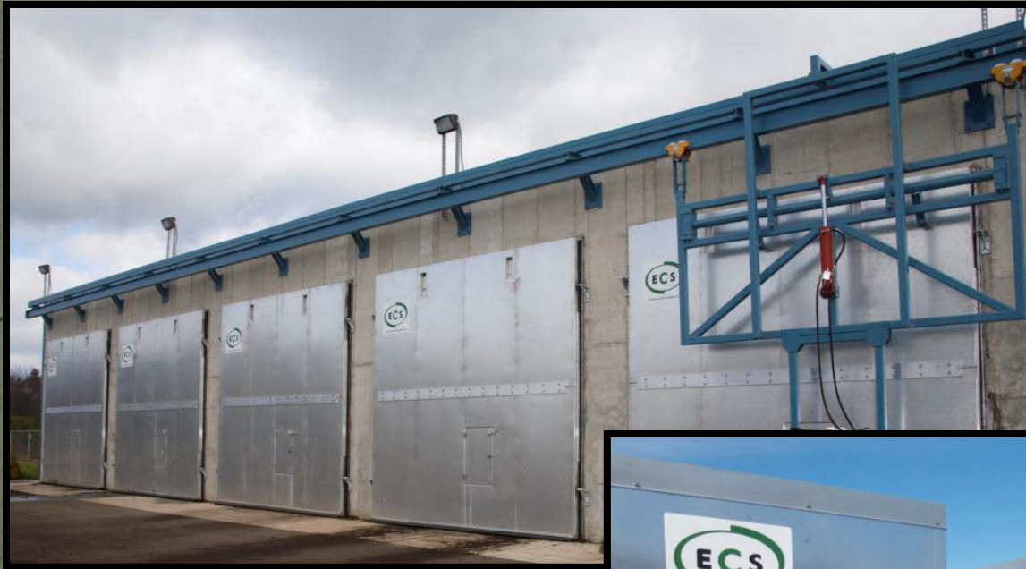
ISHPEMING, MI WTP BIOSOLIDS COMPOSTING
