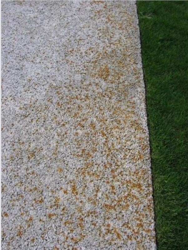
Staining from compost spilling onto pervious concrete.
