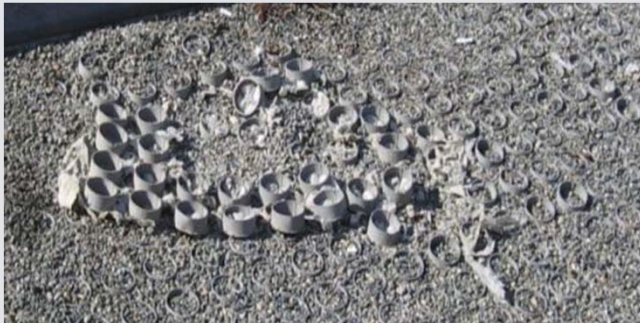
Not installed per manufacturer requirements?
