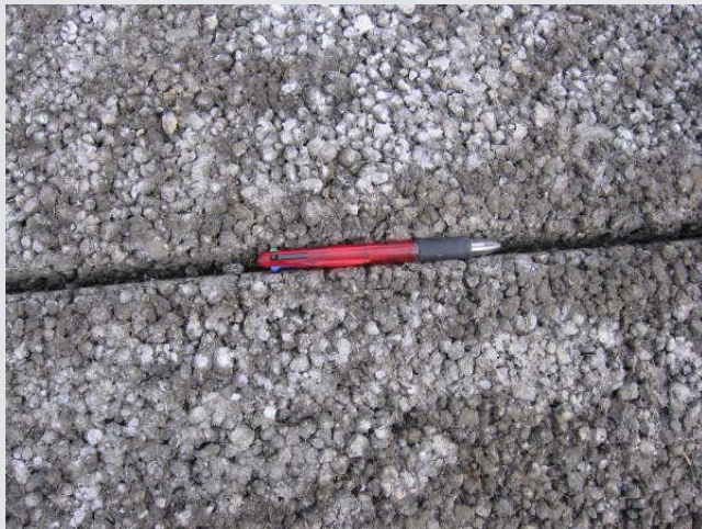
Too wide tooled joint
