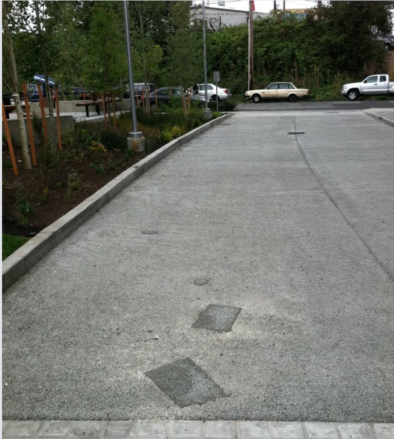
Patching due to footprint indentation.
