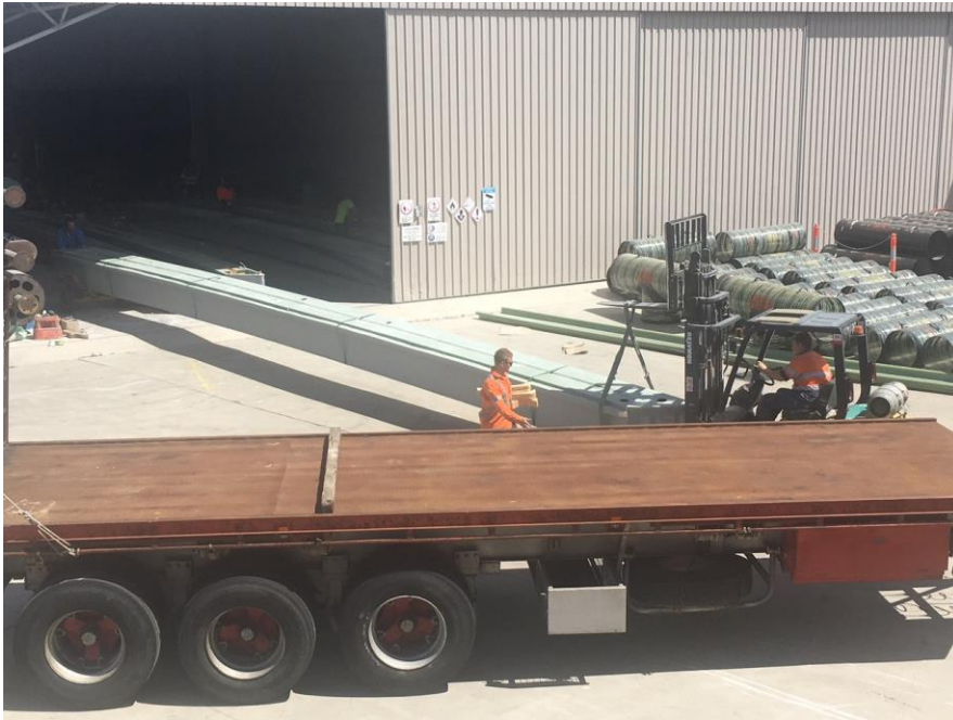
Figure 7. Typical HCB unit for Bridge 2 – West Street, Greta, being loaded on truck with forklift.
