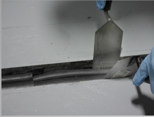
Loosen damaged material
