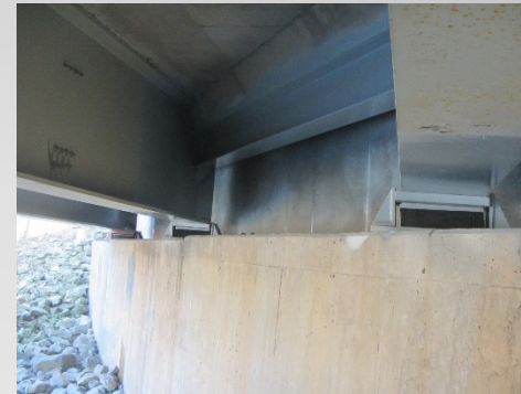
No leaks after 2 ½ years
