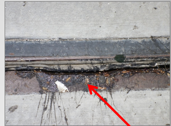
Wax emulsion bleeding during hot weather
