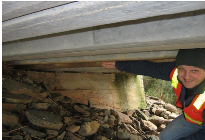
Figure 3. Picture of the author during a closer inspection where discrepancies in u-slab beam levels due were immediately obvious and due to abutment subsidence on the main bridge.
