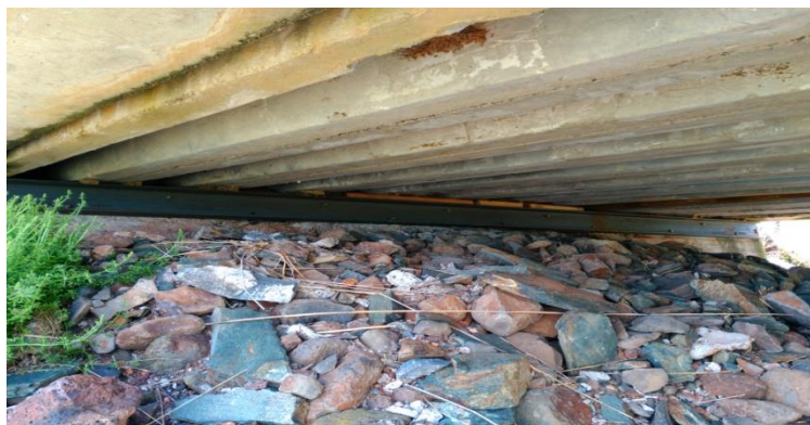
Figure 5. Steel c-section bolted through to the abutment, bracing it and preventing further subsidence
