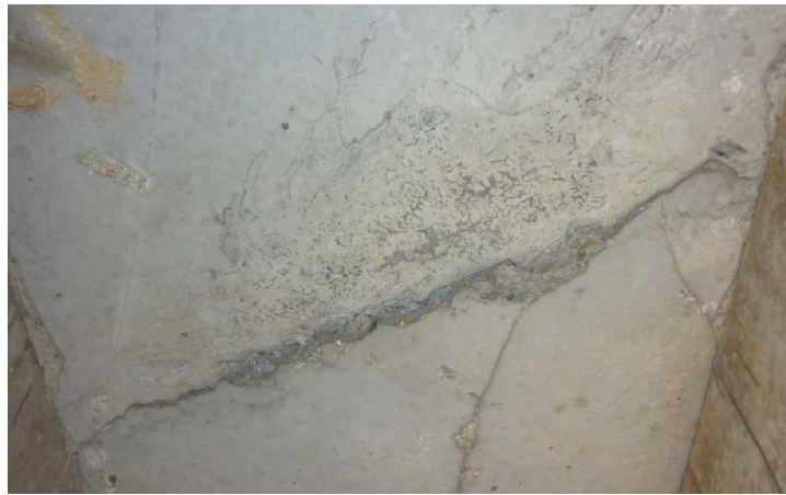
Figure 8 Deck soffit construction defect
