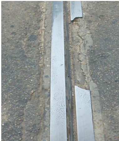
Figure 7 Deck joint failure
