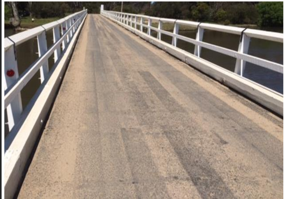
Image 8: Boundary Rd Bridge mid BRP Installation & BRP Road Patch 1 year post installation July 2017
